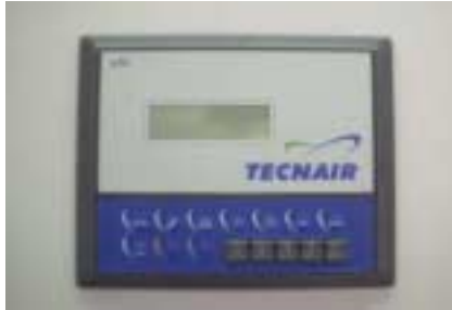
Installed on the unit
