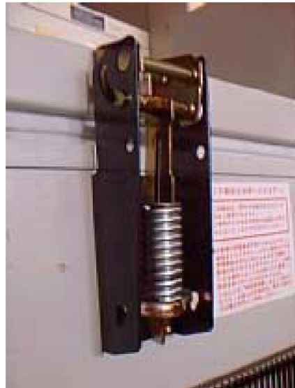
Door hinge cover removed
