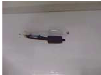
Temperature control sensor (Loaded)
