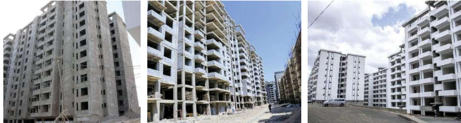
Gurd Shola, Ethiopia Project: Noah Garden Apartment Type: Residential Year: 2018 Product: Multilayer Plumbing System
