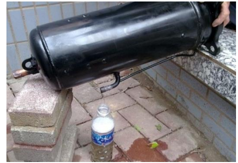
Figure 6-2.5: Draining oil from a compressor
