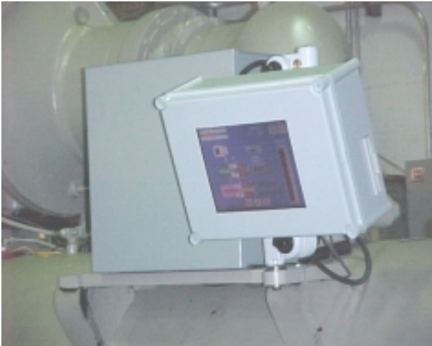
Figure 1, Unit Controller and Operator Interface Touch Screen
