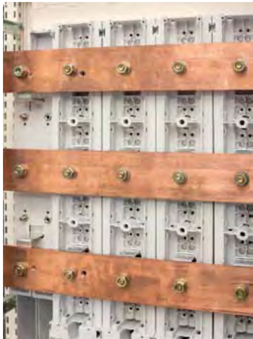
ISFL250 (direct connection on 185 mm 2 busbar).
