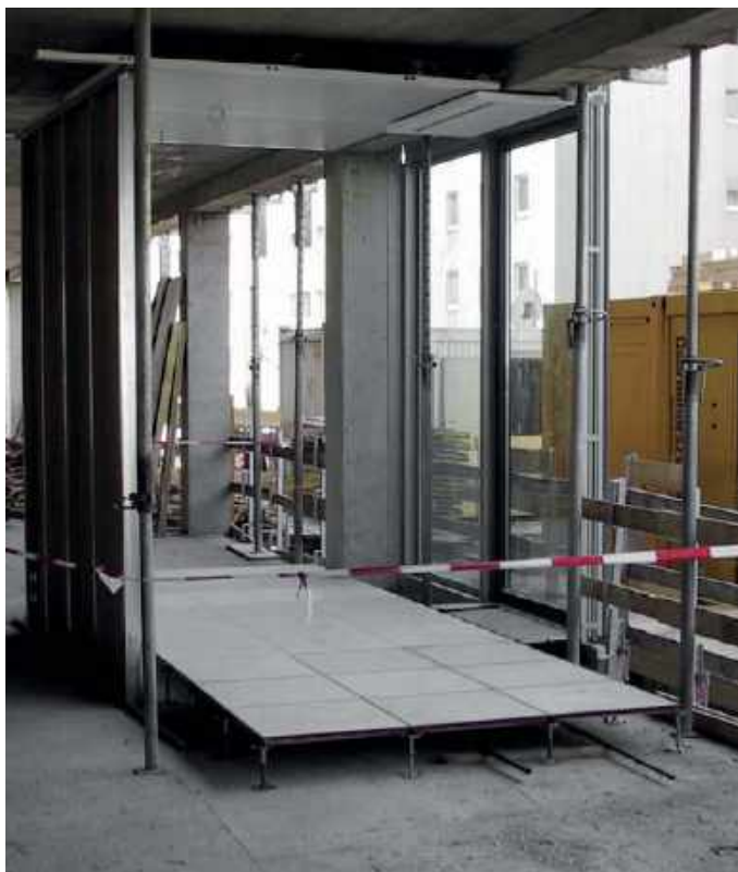
Model installation - functionality verification
