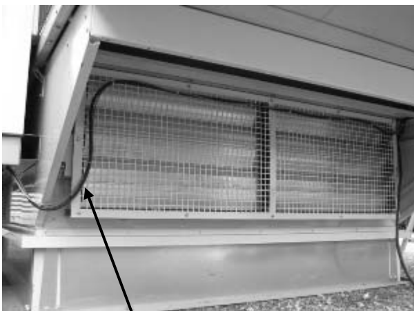
Energy recovery cable fixed on the grid of the roofcurb
