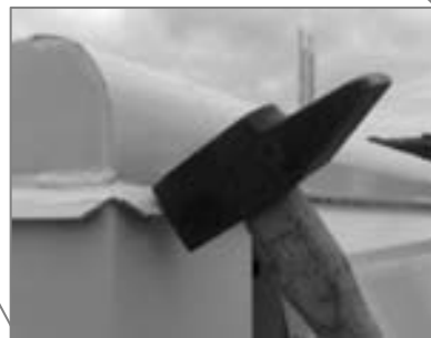
The head guard on the left corner of the rooftop has to be flattened.
