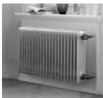
Before: Old radiator
