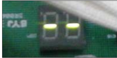
PIC 3: Main board LED when power on and unit standby.
