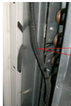
After being reconnected, the system becomes normal
