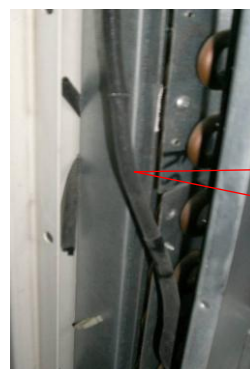
After being reconnected, the system becomes normal
