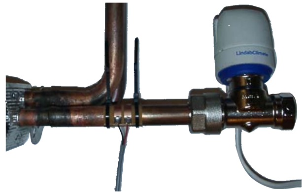
Figure 4. Sensor mounted around a horizontal, plain copper pipe and secured with two stripes
