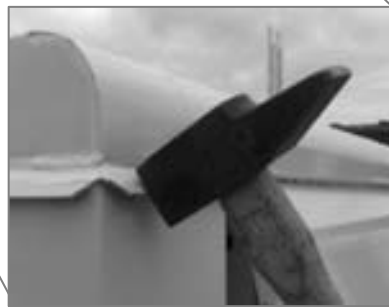
The head guard on the left corner of the rooftop has to be flattened.
