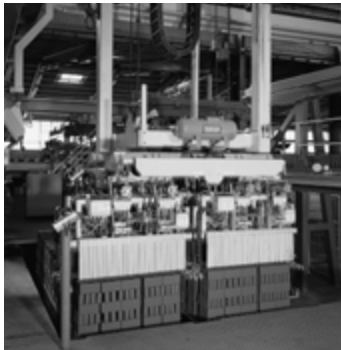
Stainless steel flexible tubes and bellows units at the kiln in the brickworks
