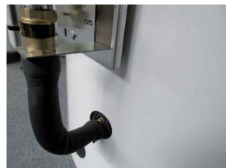
Connection at the bottom with Armaflex insulation
