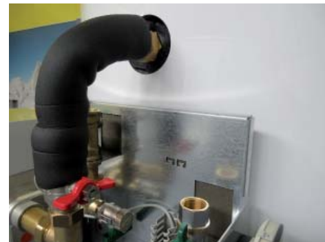
Connection at the top with Armaflex insulation
