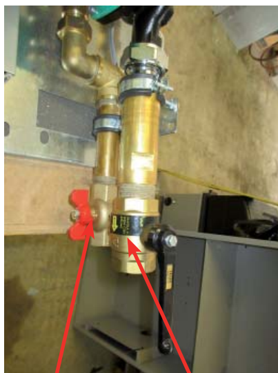
Cold water flow Tank return
