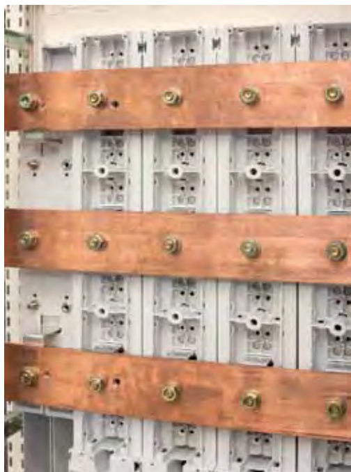
ISFL250 (direct connection on 185 mm² busbar).
