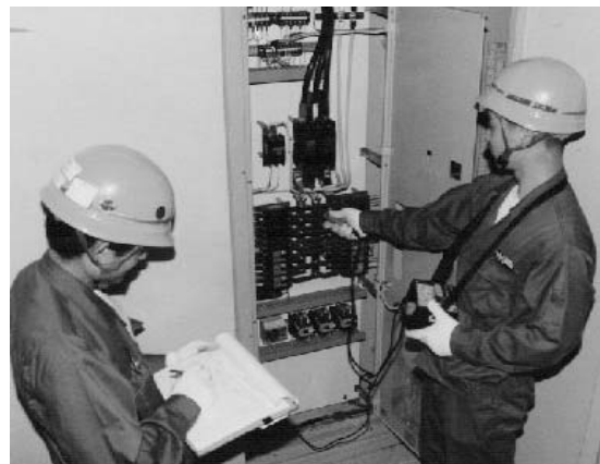
Fig. 6.12 Measuring insulation and power supply voltage ·check insulation with 500V insulation ohmmeter. ·Measure voltage with multimeter.
