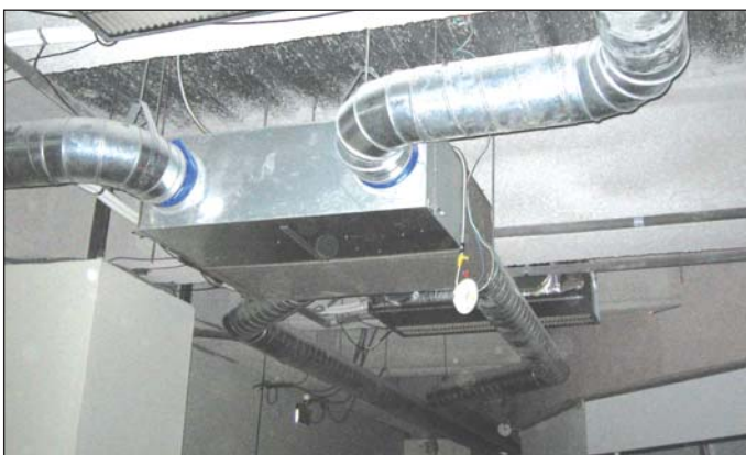
Lossnay installed in attic.
