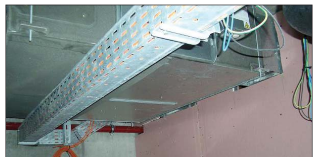
Lossnay unit is suspended from ceiling.
