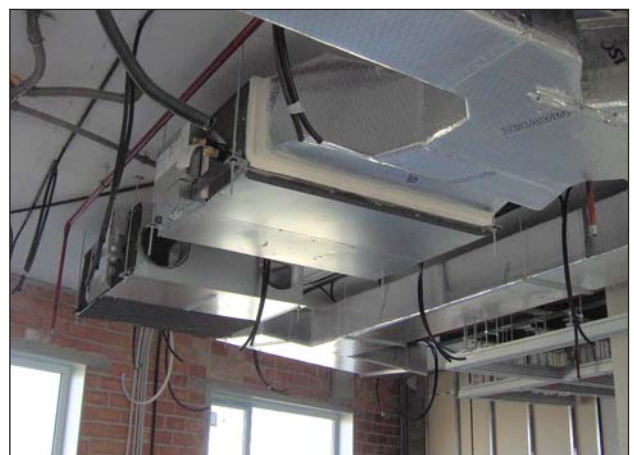
Lossnay units are suspended from ceiling.
