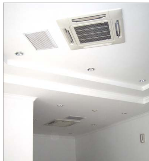
Cassette-type indoor unit installed in the ceiling.
