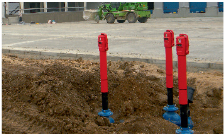
AVK series 34/00 post indicators for fire protection at FM Logistics - Petresti, Romania.
